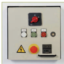
Detail of control panel with piece counter
